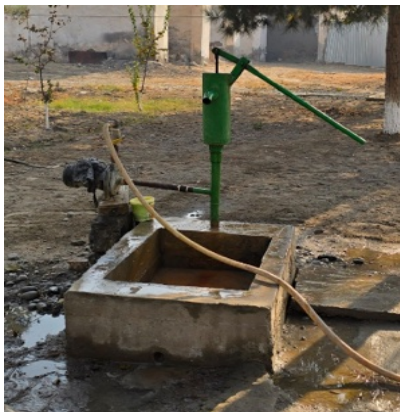
Photo 1. On-site well in Farkhor SES
