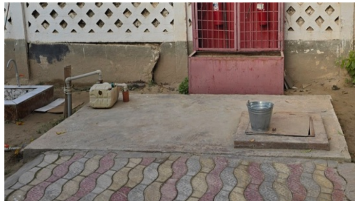
Photo 2. Jayhun SES, an underground water storage tank
